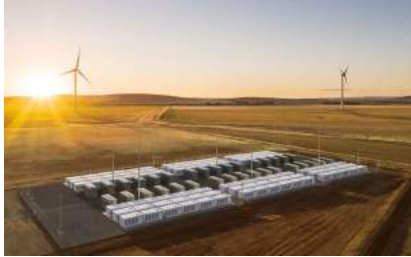
(写真) The Hornsdale Power Reserve https://hornsdalepowerreserve.com.au/#
