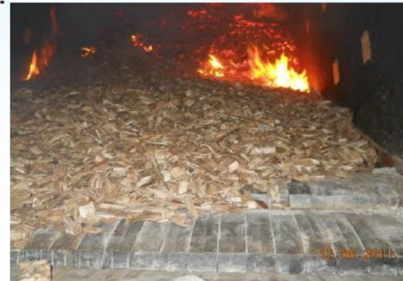
2 Biomass boilers a 10 MWh
